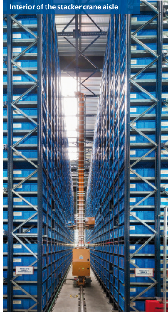
Access doors to the stacker cranes
