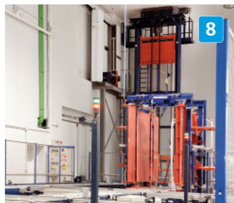
The roller or chain conveyors, automatic control station, compactor, lifts and security features all ensure an automatic, secure and high-capacity transport control.
