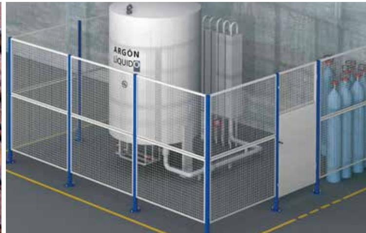
Chemical products area
